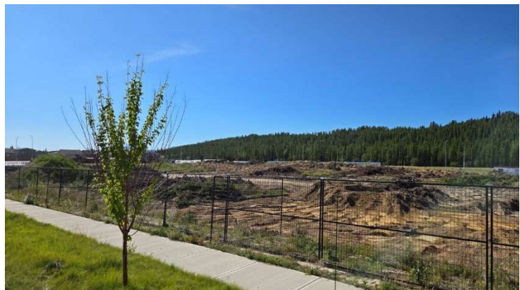
Trees have been removed from the Whistle Bend site and ground is being prepared for grading and preloading.
